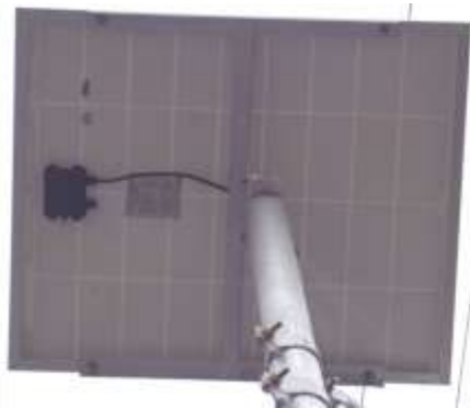
Fig.2.4: Solar Module Back Side
